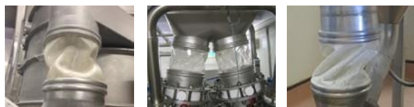
Installation gap too small
